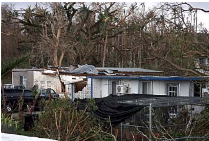
Housing damage on Guam from Super Typhoon Pongsona
