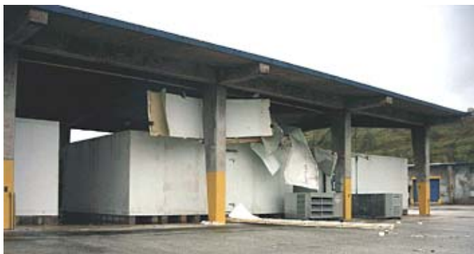
Reefer 4 damage rear view.
